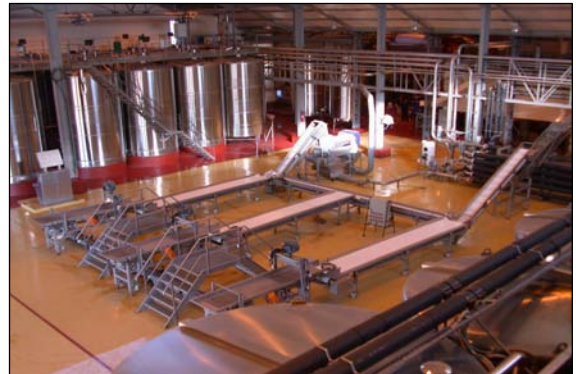
Celliers de Meknès (Morocco) : manual reception of sorted grape harvest capacity 30 tonnes/hour.
